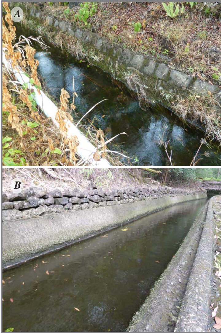
Figure 5. Photographs of two sections of the Ko'olau Ditch, East Maui Irrigation diversion system, east Maui, Hawai'i. A , Lined open-ditch section near Makapipi Stream with armored cut-stone walls and concrete bottom. B , Lined open-ditch section near Waiohue Stream with concrete walls and bottom.
