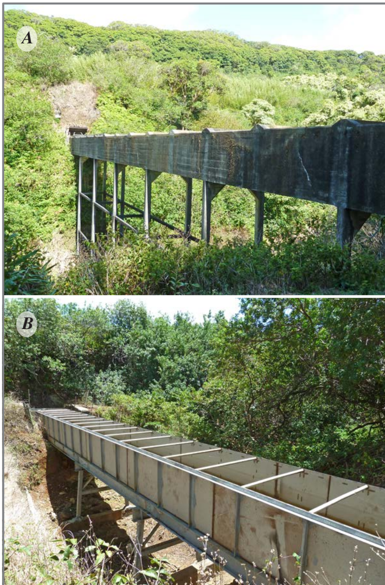
Figure 4. Photographs of two flumes that are part of the East Maui Irrigation diversion system, east Maui, Hawai'i. A , Concrete-lined flume along the Wailoa Ditch at 'Ōpana. B , Stainless-steel flume along the Lowrie Ditch near Kuiaha Gulch, also known as Labasan flume.
