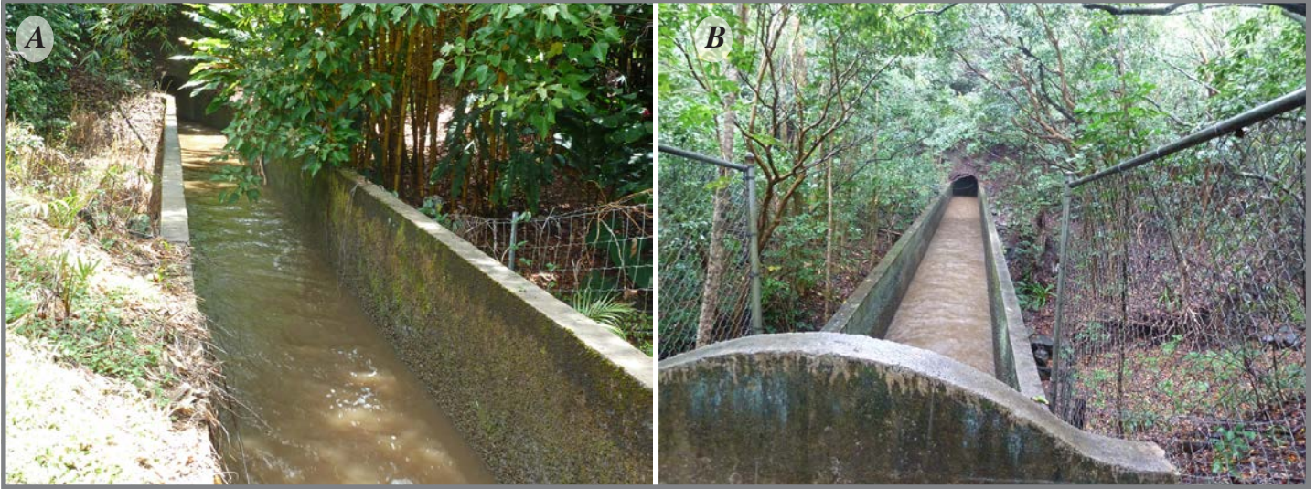
Figure 10. Photographs of two sections of the Ha'ikū Ditch, East Maui Irrigation diversion system, east Maui, Hawai'i. A , Eby Flume at Manawaiiao Stream. B , Shiota Flume at Kuiaha Gulch.
